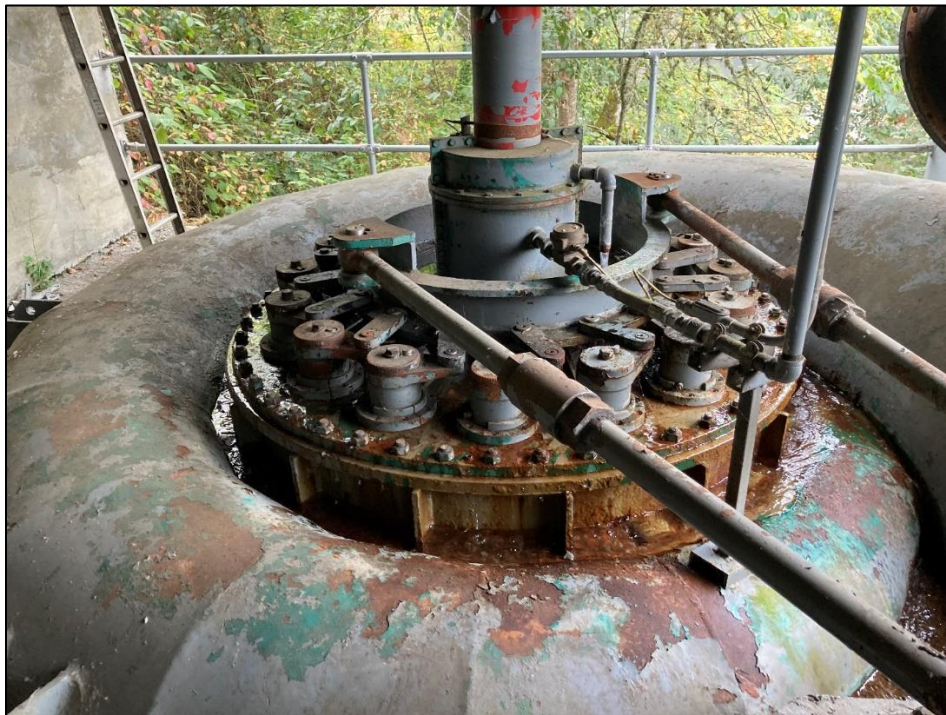
Figure 7-2. Hydroelectric Scroll Case and Wicket Gates Photo
