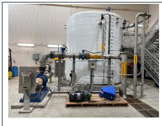
Photo 22 AM – Clean-in-Place Tank and Pump
