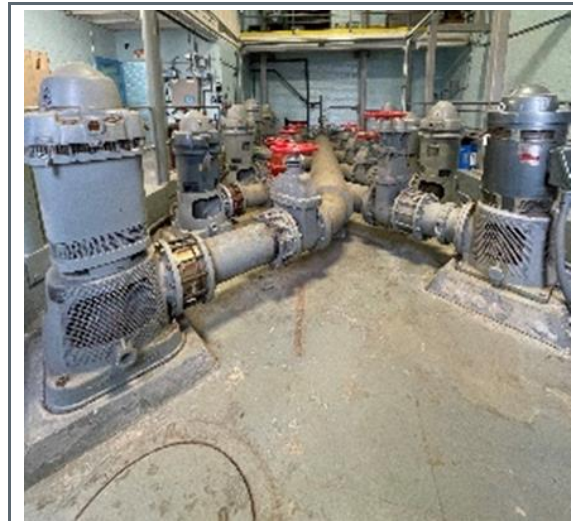
Photo 3 Vine Street – Raw Water Pump Station Interior
