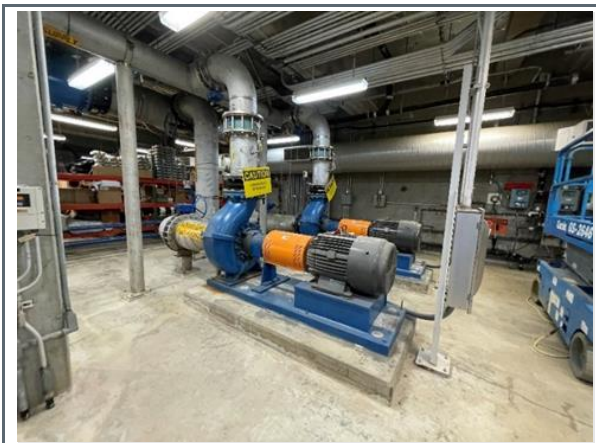
Photo 20 AM – Backwash Pumps
