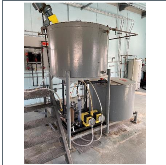
Photo 5 Vine Street – Dry Chemical Room
