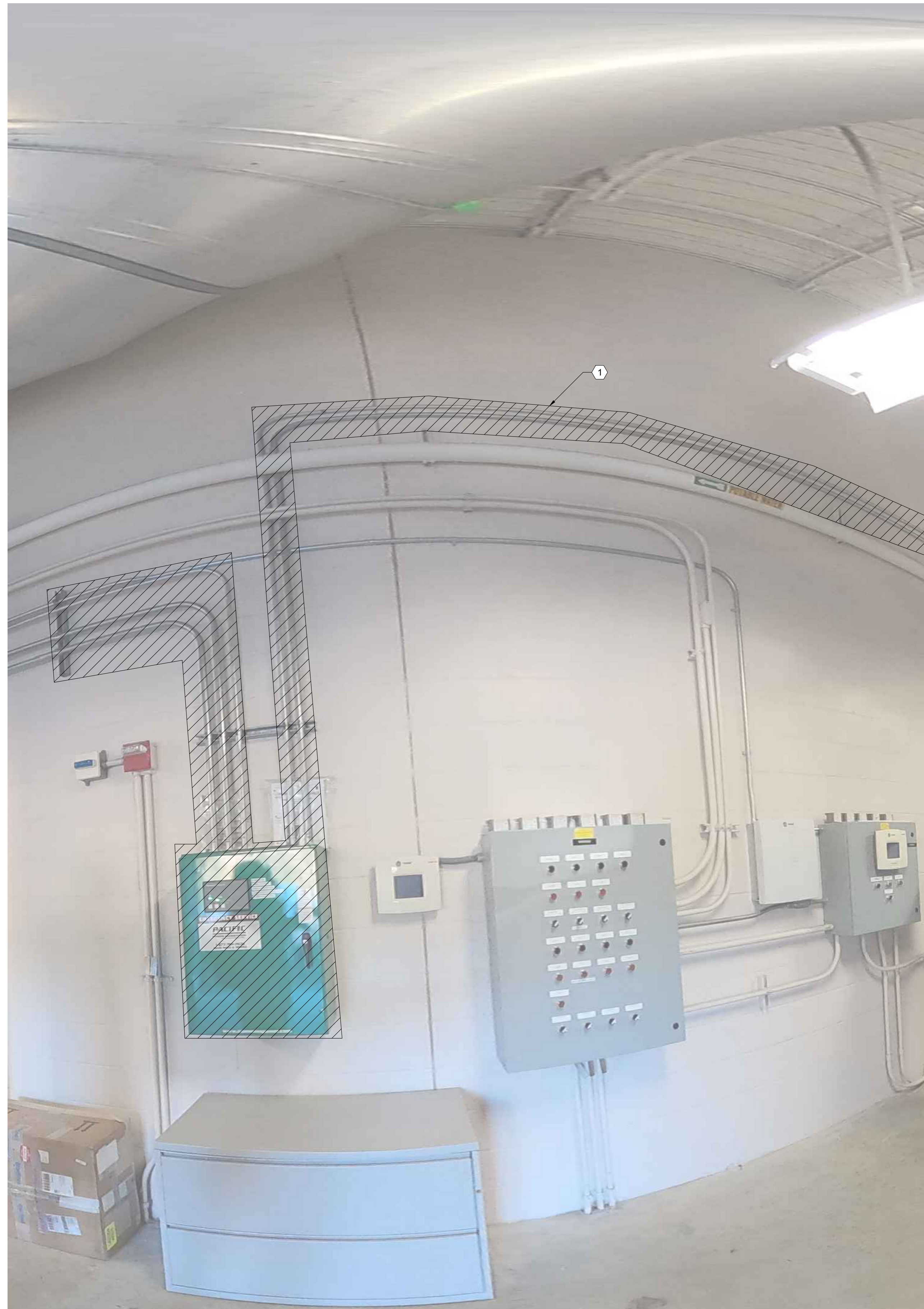
1 ELECTRICAL DETAIL PHOTO SCALE: NTS
