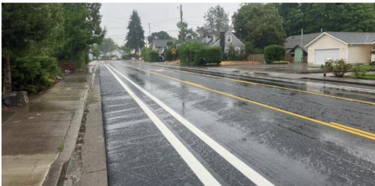
Queen Avenue shown after reconstruction, restriped to create a bicycle lane buffer on this heavily traveled street that fronts a large middle school and a large high school.
